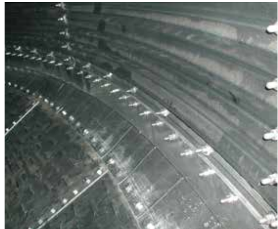
— Photo of FCV28 inside the silo
